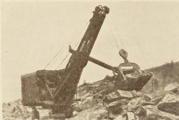
FIGURE 7.—SHALLOW CUTS IN HARD ROCK ALWAYS PROVE EXPENSIVE. ALTHOUGH THE CONTRACTOR SPENT $2 PER CUBIC YARD ON DRILLING AND BLASTING IN THIS CUT (MOSTLY 2 TO 4 FEET DEEP), THE ROCK WAS STILL SO POORLY BROKEN THAT THE COST OF GETTING IT INTO THE FILL ADDED OVER ANOTHER DOLLAR
